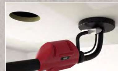
D / Sand joints only Sand the filled joints with your preferred tool to level the panel surface.
