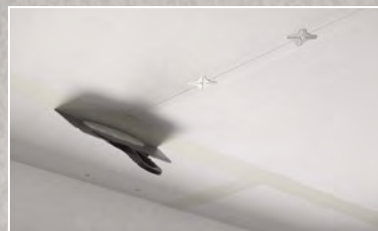
C / Fill joints, insert tape and finish joints Use your preferred tool to fill the joint. Repeat until the joint is properly filled.
